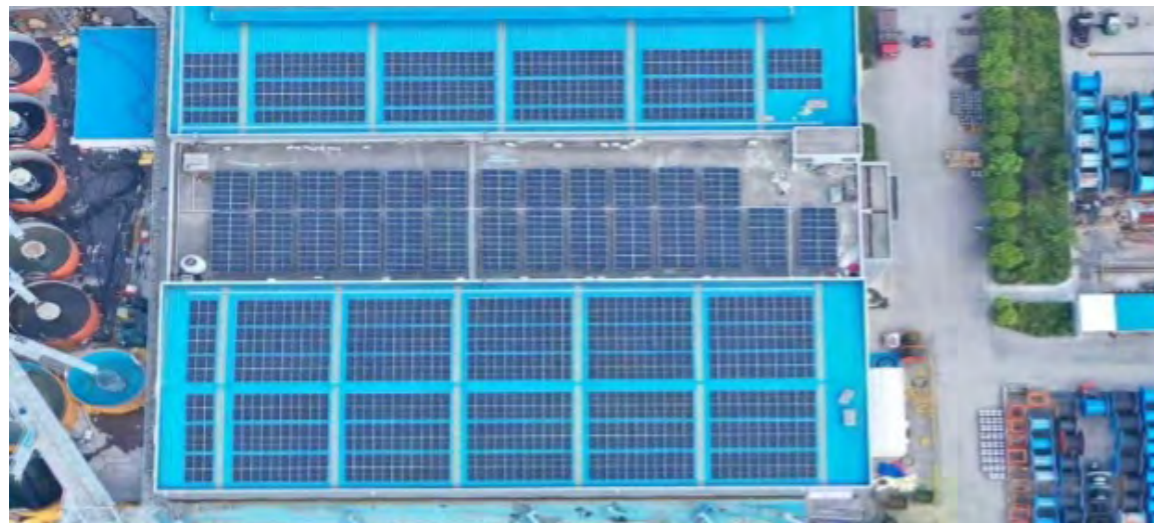
Jiangsu Hengtong Huahai Technology Co., Ltd. Self-Built Photovoltaic Project
